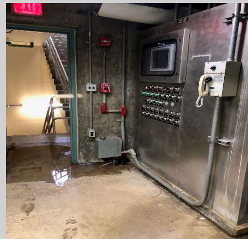
Oxygen Reactor Controls and Electrical Systems
