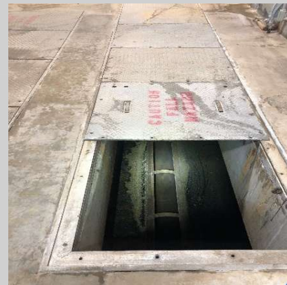
Secondary Rotating Scum Pipes Access
