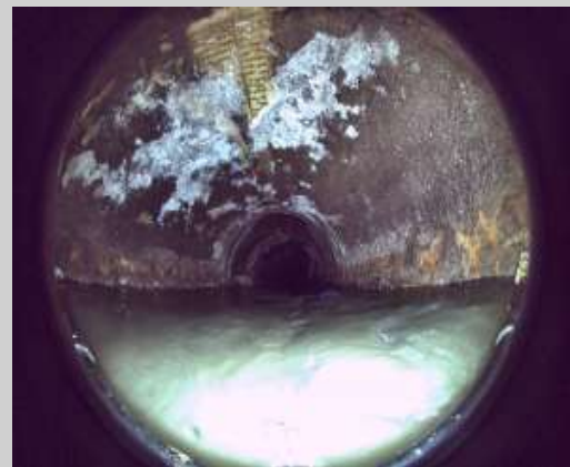
84-inch RCP showing Corrosion and Deposits
