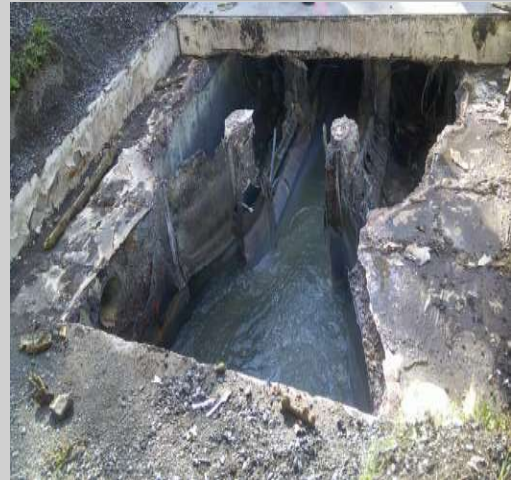
Bass River Upstream Siphon Chamber With Removable Precast Planks Removed
