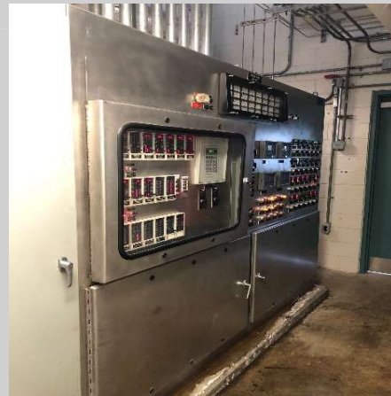
Oxygen Reactor Control Panel
