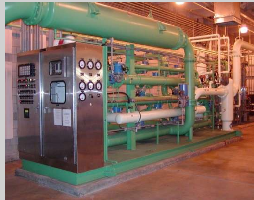
Oxygen Generation Process Equipment
