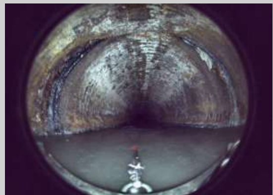
54-inch Reinforced Concrete Pipe Corrosion
