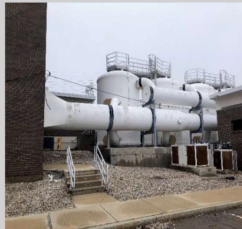
Odor G Ductwork and Activated Carbon
