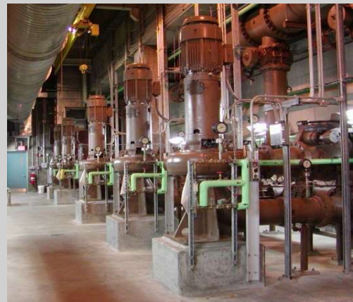
RAS Pump Gallery
