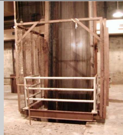
Existing bar screen with 1-inch openings
